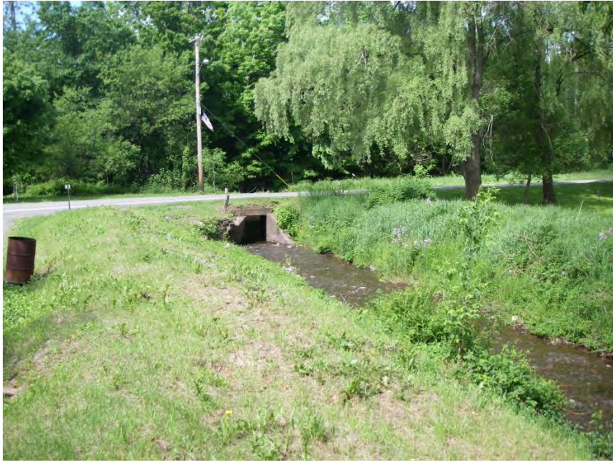
Figure 2.10 Before restoration of an undersized and failing culvert in Lexington.
