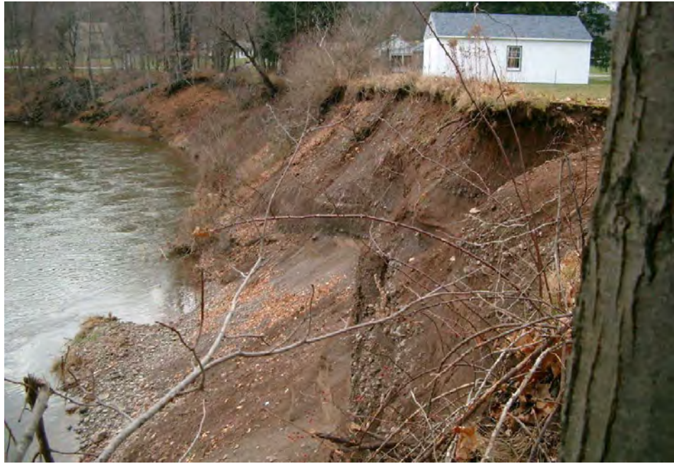
Figure 2.12 Terrace Avenue before streambank stabilization.
