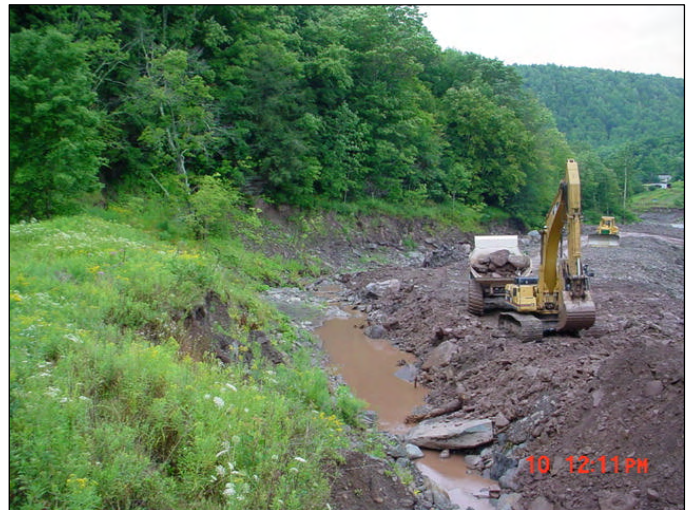
Large boulder materials being salvaged before filling of the upstream high bank.
