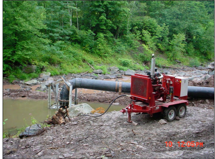
Phase I dewatering pump intake and pipeline.
