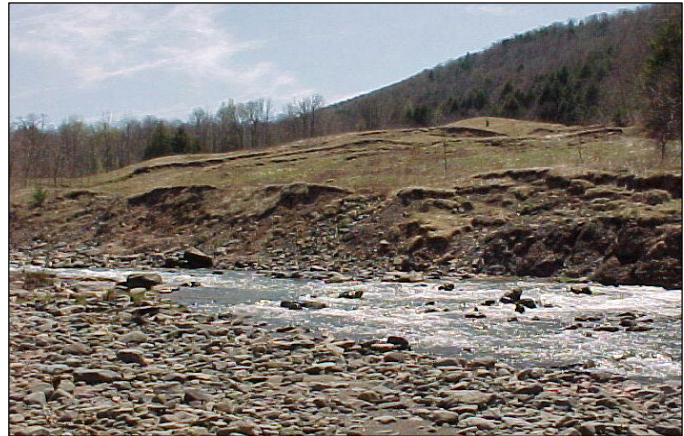
Erosion and failure of upstream high bank in 2001.
