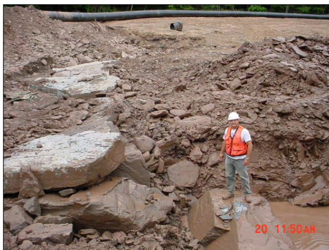
Excavation and construction of a cross vane sill near the center of project reach.
