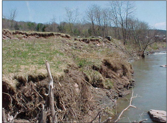
Image of downstream bank erosion and failure.
