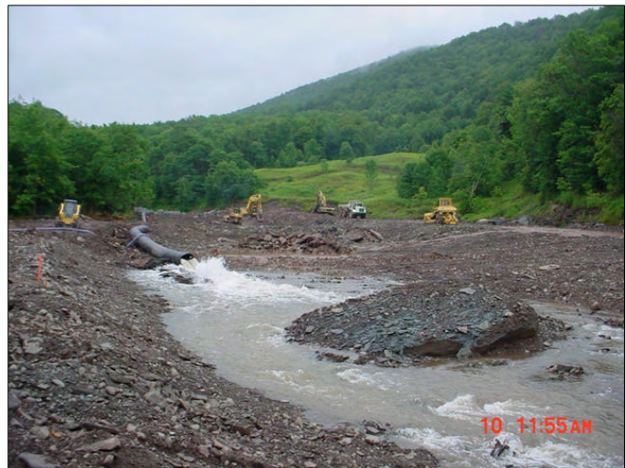
Phase I dewatering outlet.
