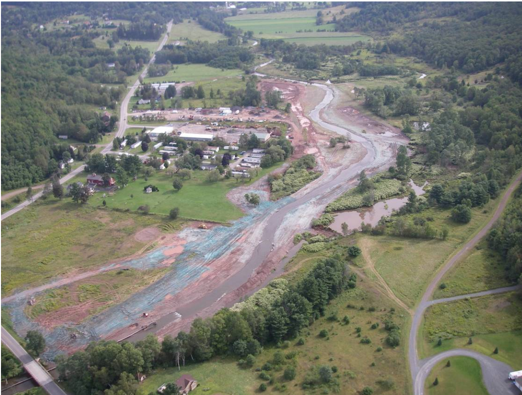
View from helicopter on September 9, 2006. Ashland project in foreground with Brandwyne project in background.
