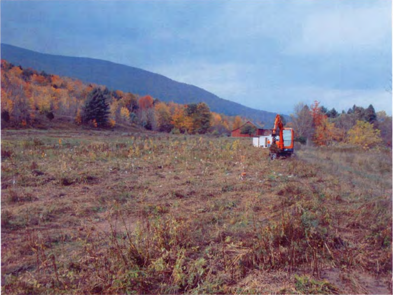
Figure 2: GCSWCD staff planting containerized trees and shrubs along left floodplain west (downstream) of the Carr Rad Bridge. Each white spot represents a plants label. The excavator with hydraulic auger facilitates planting in the rock soils characteristic of the Schoharie floodplain.
