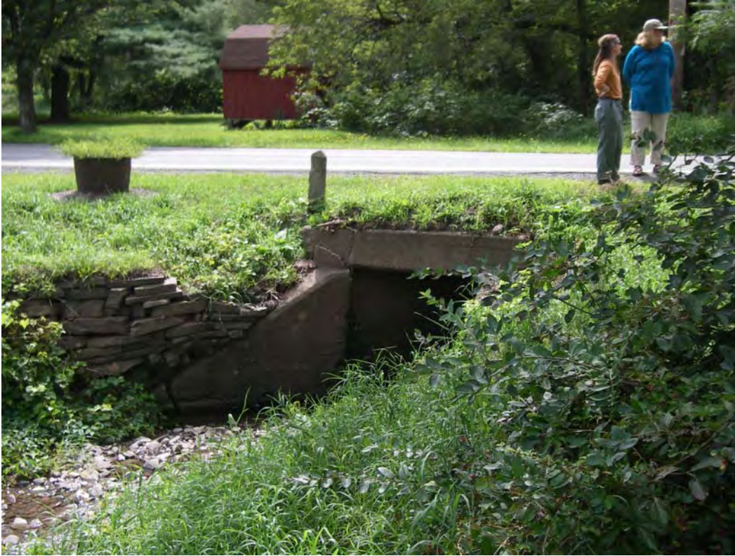
Photo 1: View looking downstream at entrance to existing concrete culvert. Note failed headwall.
