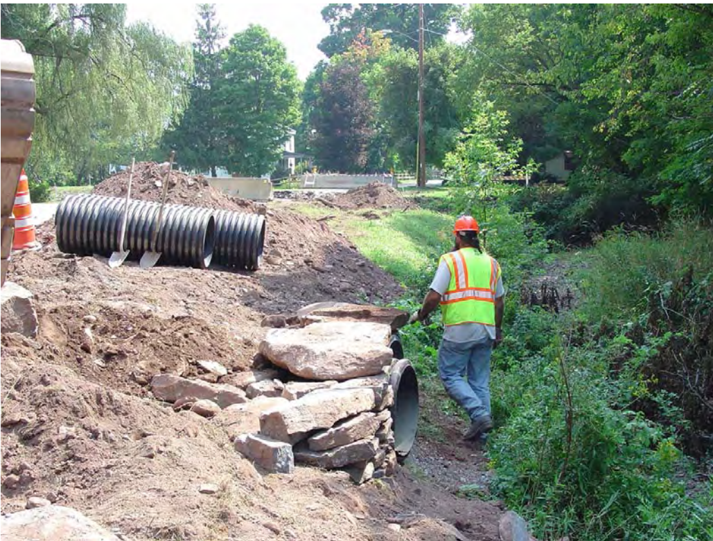
Photo 4: Laid up headwall on outlet of floodplain drains. Invert has been set high on the bank to allow discharge at flood stage.
