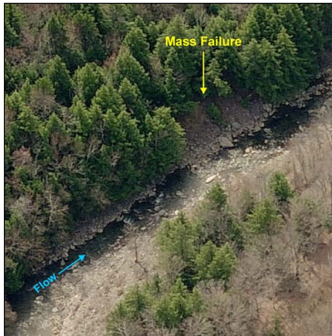
Bank erosion at Station 120200
