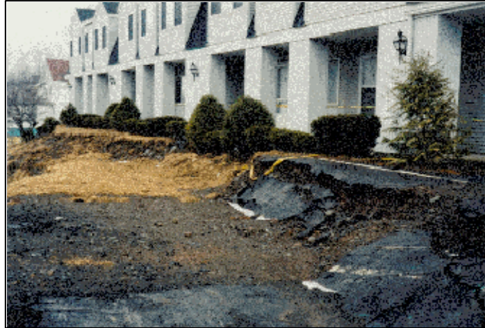
Melody Woods Complex after 1996 flood event (Station 109900-109350)
