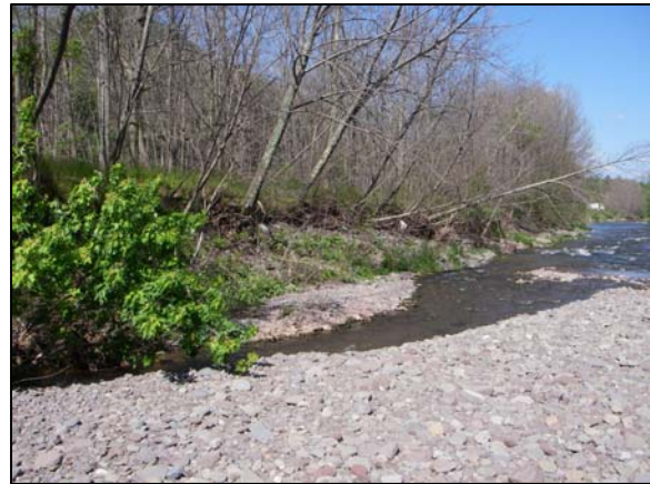
Bank erosion at Station 108100
