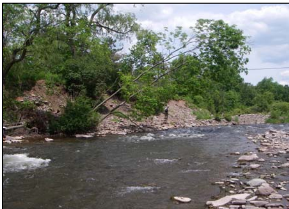
Bank erosion at Station 99700 - looking upstream
