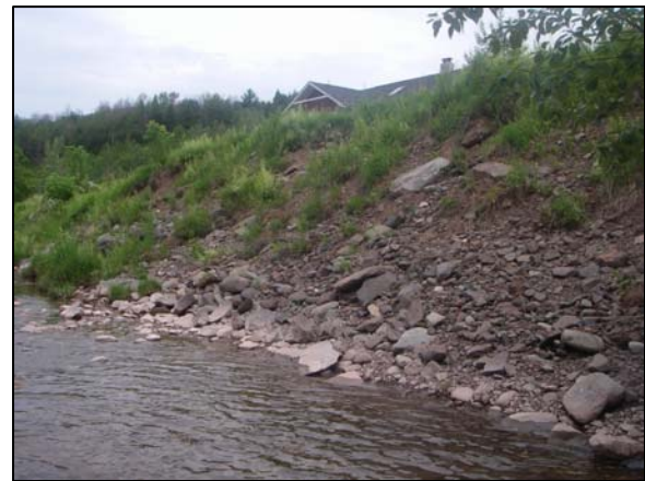
Bank erosion and planting site at Station 88000
