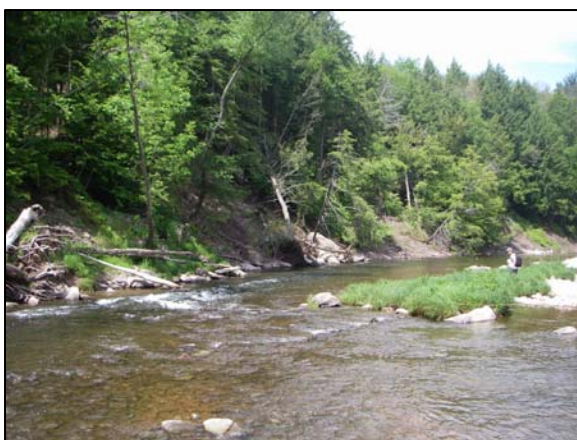
Bank erosion at Station 73100
