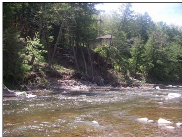
Bank erosion at 78900
