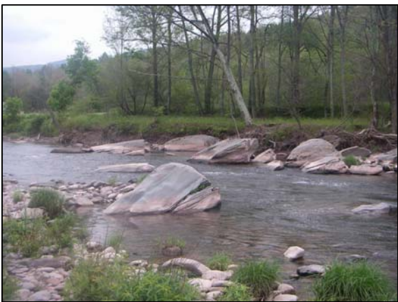
Bank erosion at Station 67300 - looking upstream
