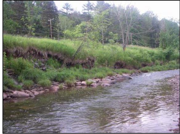
Bank erosion at Station 69050
