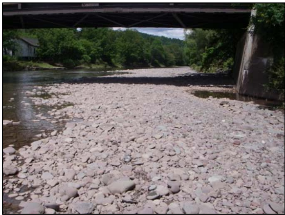
Aggradation at County Route 42 bridge Station 55350
