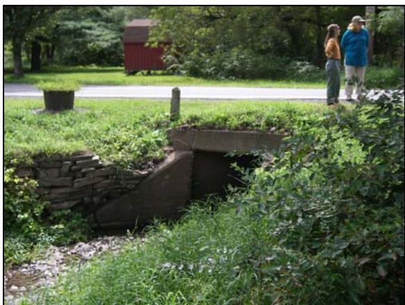
Culvert in need of replacement on County Rt. 13A
