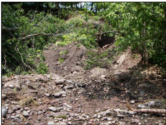
Bank erosion at Station 45560
