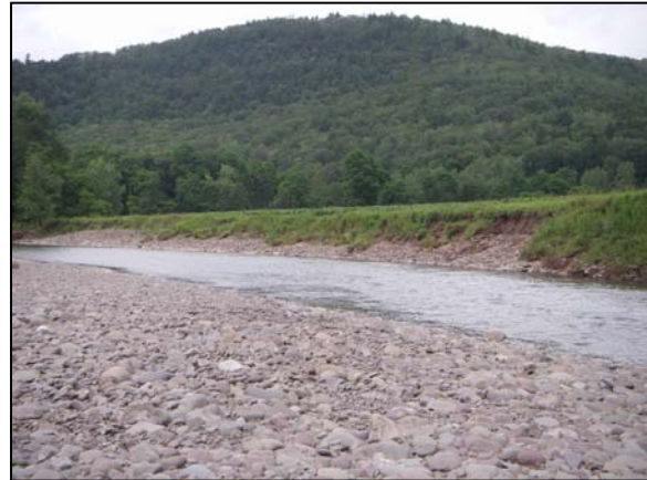
Bank erosion at Station 20300
