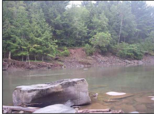
Bank erosion at Station 26260
