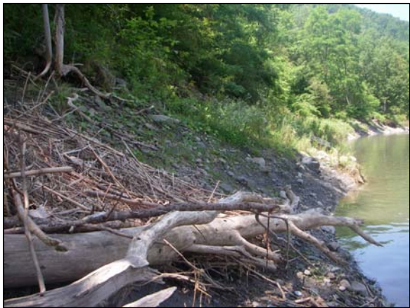
Bank erosion at Station 13650
