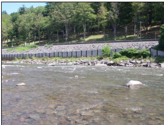
Revetment at Station 16400
