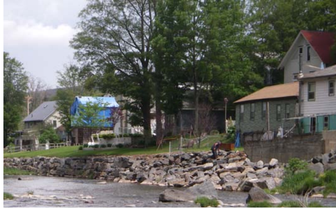
Streamside development and mowing to the edge of the stream leads to bank failure. This bank has been reinforced with riprap and concrete.
