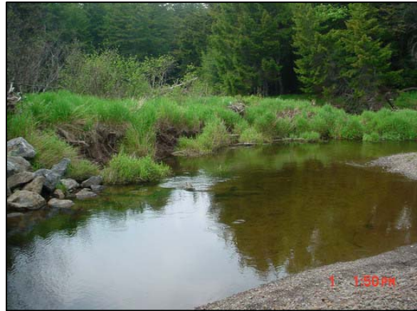
Bank erosion and clay exposure at Station 148200
