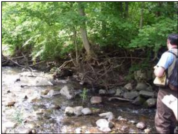
Erosion at Stations 21520 - 21386
