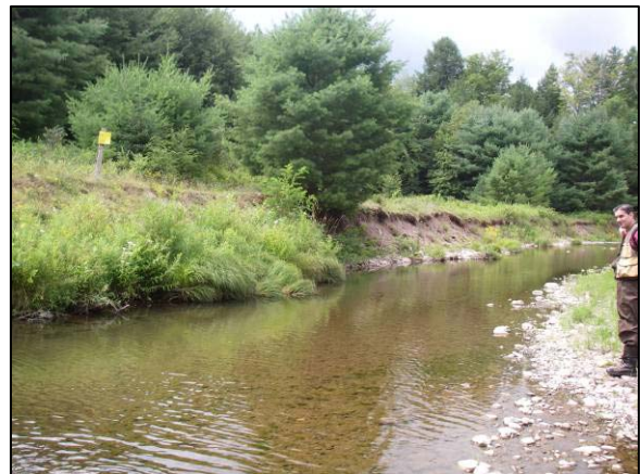
Erosion at Stations 19405 - 19009
