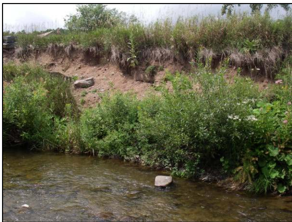
Erosion at Stations 17200 - 17010
