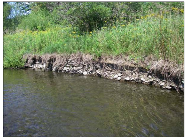
Erosion at approximate Stations 13050-12960
