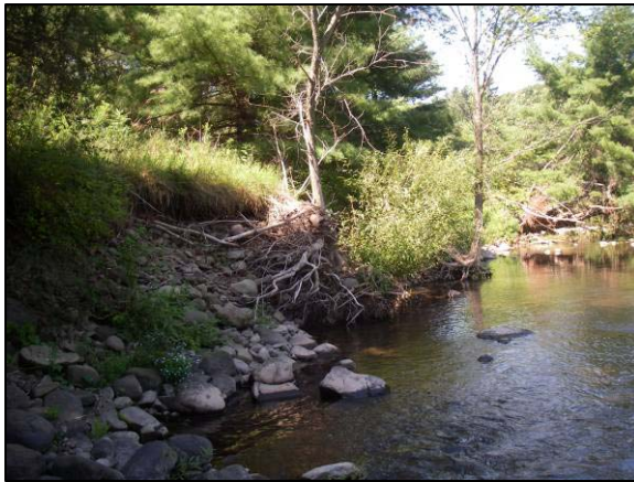
Erosion at Stations 10630-10266
