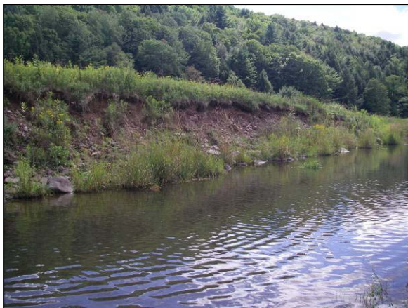
Erosion at Stations 14180 - 14043
