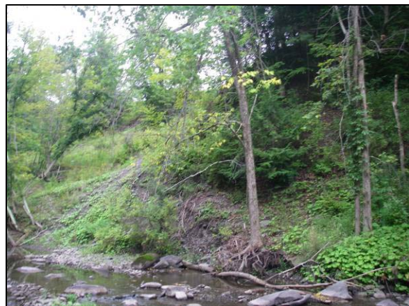
Mass Failure at Stations 8123-7800
