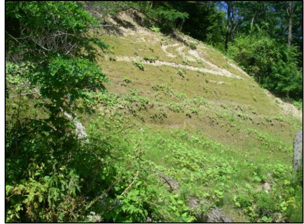
Mass Failure at Stations 2552-2411
