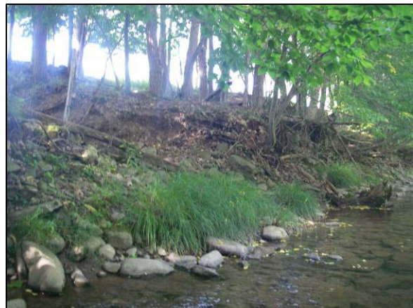
Erosion at Station 4304
