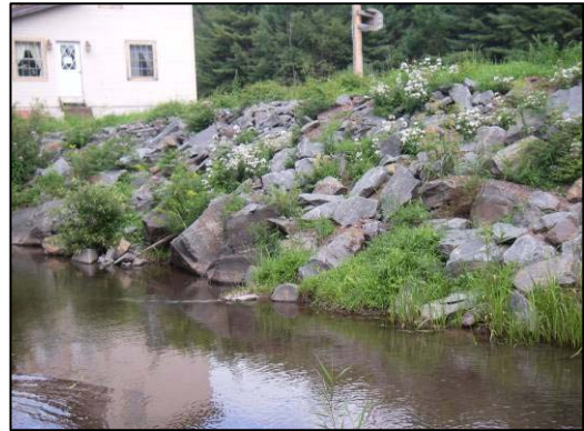
Streamside development and limited riparian vegetation leads to compromised streambanks. This bank has been reinforced with riprap.
