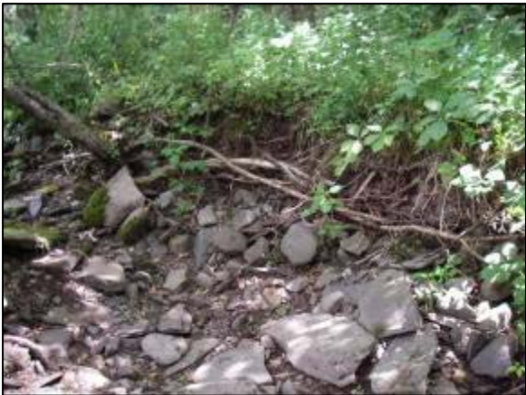
Eroding bank, Stations 48259 -48181
