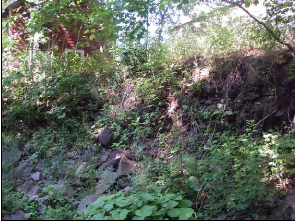
Erosion at Stations 42216 - 42164
