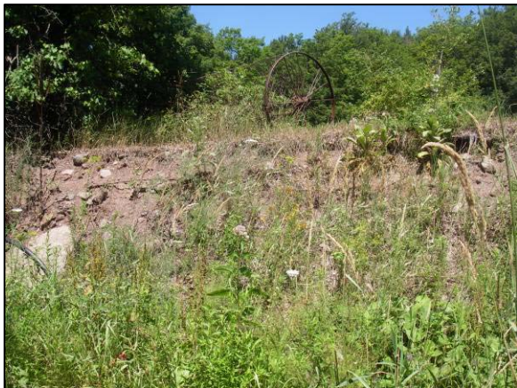
Erosion at Stations 40950 - 40787
