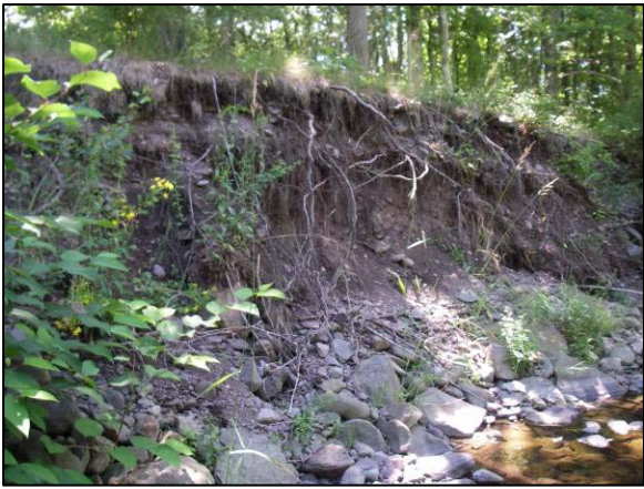
Erosion at Stations 42815 - 42692
