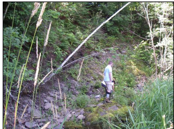
Erosion at Stations 45083 - 44941
