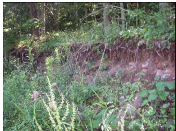
Erosion at Stations 41805 - 41651
