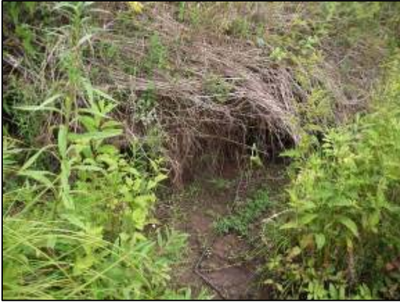
Erosion at Stations 28600 - 28585
