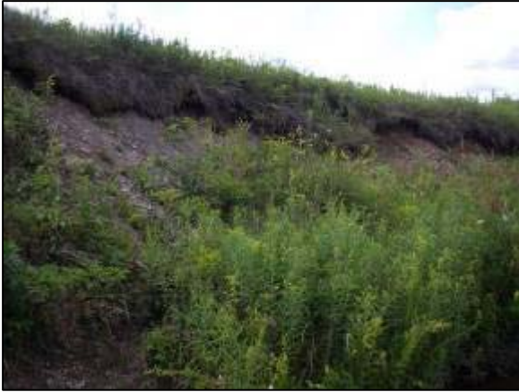
Erosion at Stations 29319 - 29201
