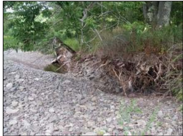
Erosion at Stations 36800 - 36580
