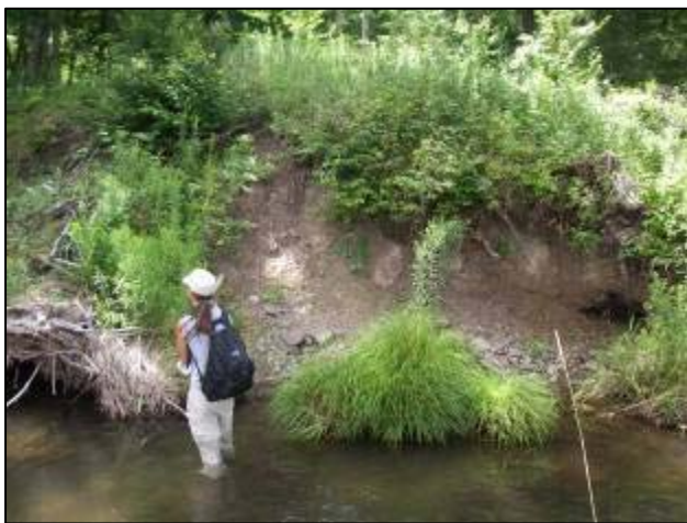
Erosion at Stations 30011 - 29959
