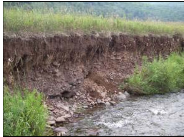
Erosion at Stations 34100 - 33881
