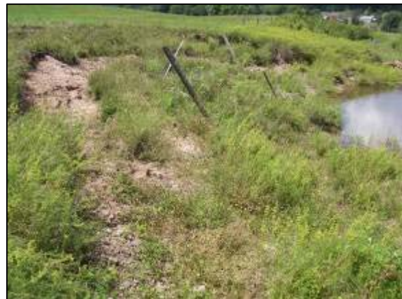
Mass Failure at Stations 29682 - 29664
