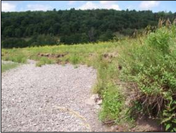
Erosion at Stations 36183 - 34909
