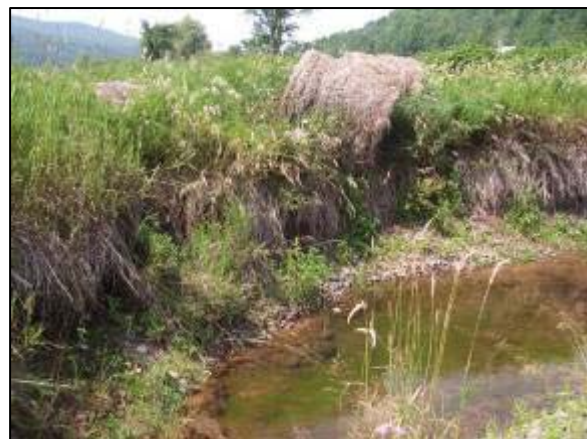
Erosion at Stations 34658 - 34547
