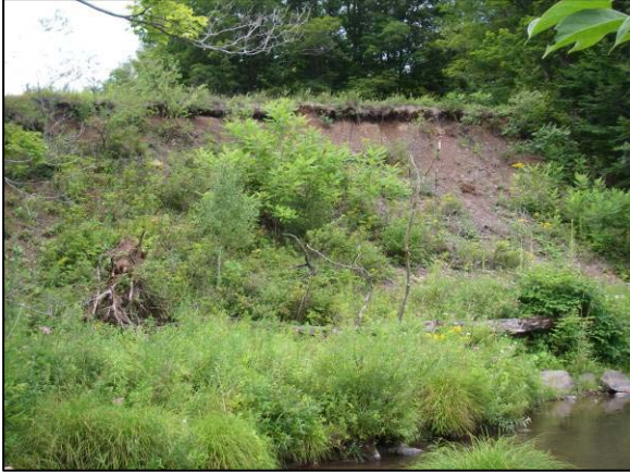
Mass Failure at Stations 27163 - 26938
