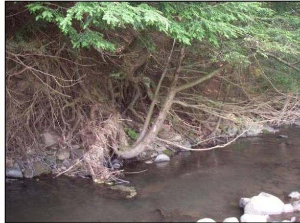
Erosion at Stations 25098 - 24981
