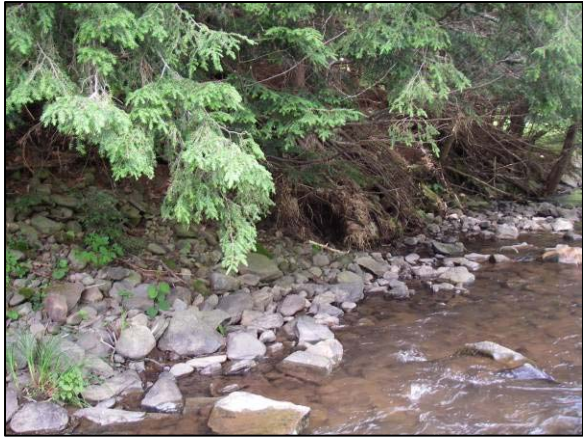
Erosion at Stations 26588 - 26432
