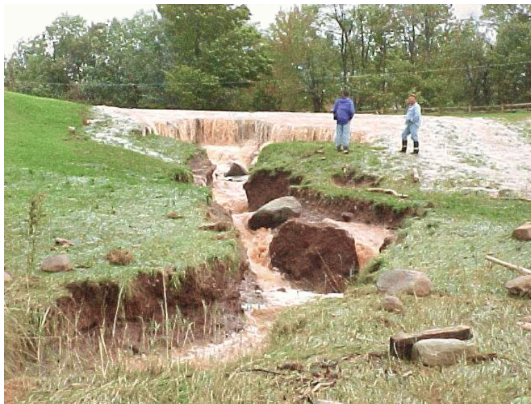
Figure IV-47: Damage to north emergency spillway on the C.D.Lane dam as the result of flows from tropical storm Floyd reduced.
