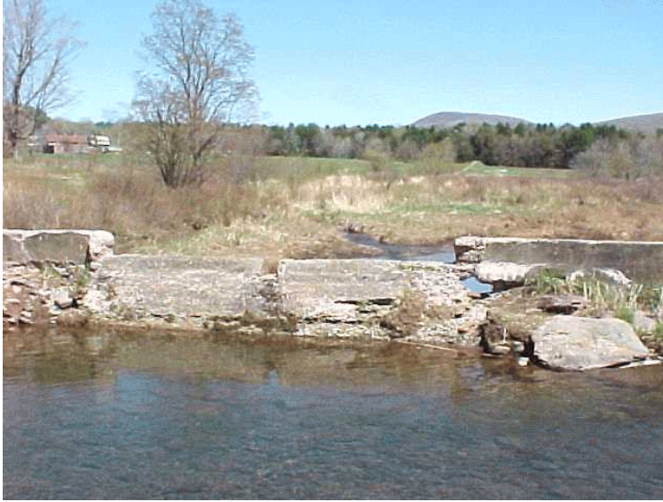
Figure V-39: Concrete dam presents a fisheries migration barrier on small tributary on the Batavia Kill.
