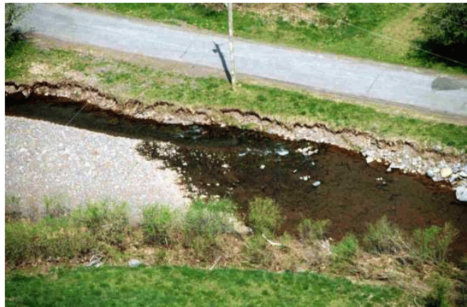
Figure VI-8: Aerial view of lateral migration along CRT in lower section of management segment 1b.
