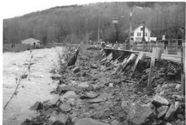
Figure VI-33: Severe streambank erosion along NYS 23 below GNH Lumber after 1961 flood.
