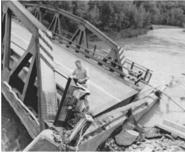
Figure VI-36: 1961 flood damage to Church Street bridge located in Reach 3c.
