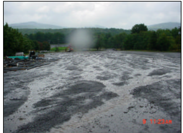
The GCSWCD is working with Windham Mountain to retrofit older development features such as this parking lot to address stormwater quality. Note the extensive rill erosion and loss of sediments.
