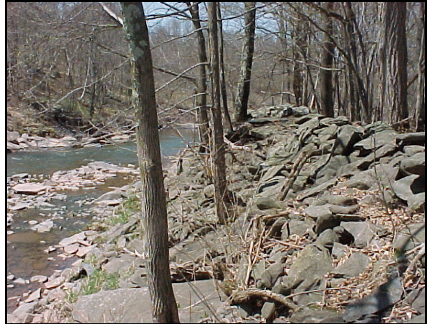
Figure VI-86: Large stone wall along right streambank increases channel entrenchment.
