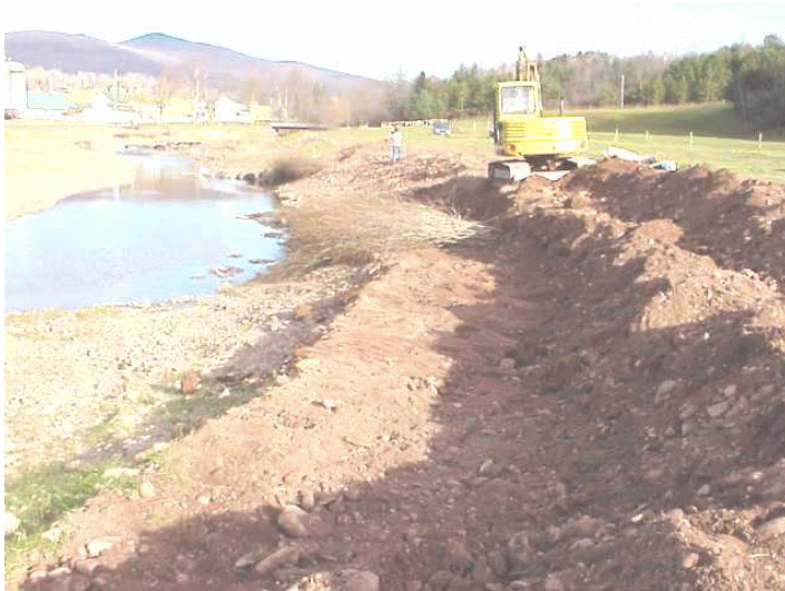
Figure III-26: Excavation of streambank benches and the placement of alternating lifts of soil and willow shoots is the basis of brush layering.
