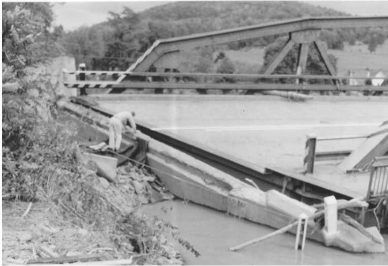
Figure IV-6: Flood damage to South Street Bridge, hamlet of Windham circa 1961.
