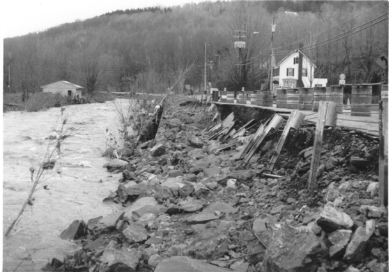
Figure IV-7: Washout of NYS Route 23 just west of GNH Lumber location.
