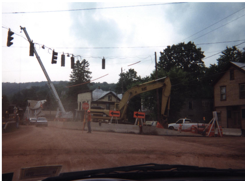
Road construction on State Highway 10 in the town of Bloomville, Cannonsville watershed.
