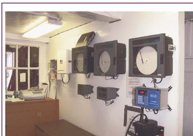
Figure 3.1 Continuous Monitoring Station at the Catskill Lower Effluent Chamber.
