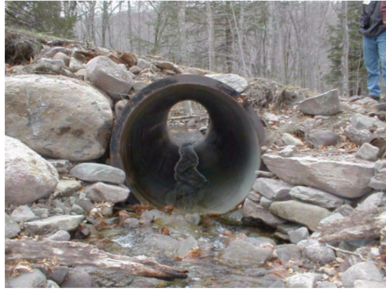
Figure 4.7 A properly installed timber harvest road culvert, a project of the Forestry Management Program, Neversink Reservoir watershed.
