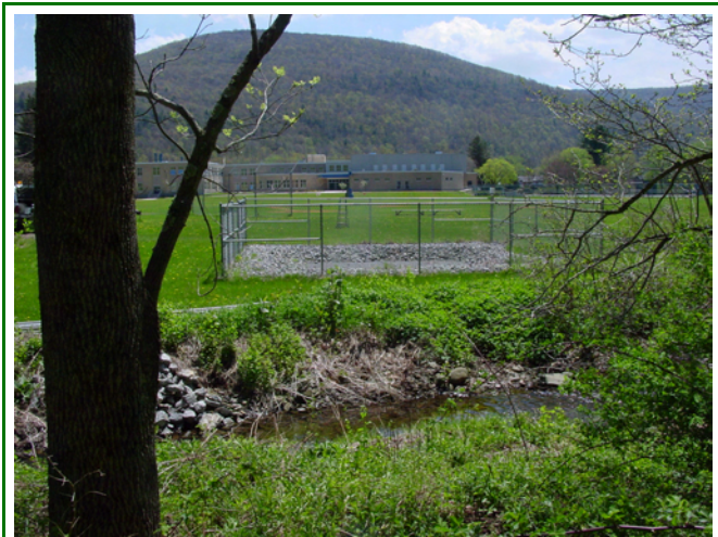
Figure 4.6 Sand filter portion of a stormwater retrofit installed at the Margaretville Central School bus garage, Pepacton Reservoir watershed.
